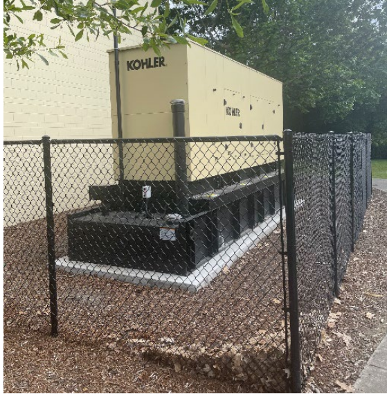
Figure 1. Generator as seen from Memorial, walkway and North Parking Lot
