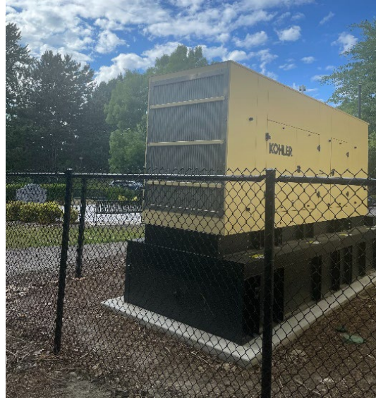
Figure 2. Generator as seen from behind, from South building walkway
